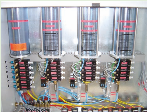
6 pumps for outside lubrication 6 pumps for inside lubrication 6 pumps for additional lubrication
